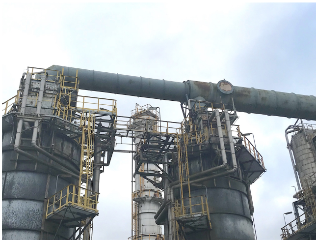
Fig. 2. Oil and Gas refinery in Germany.
